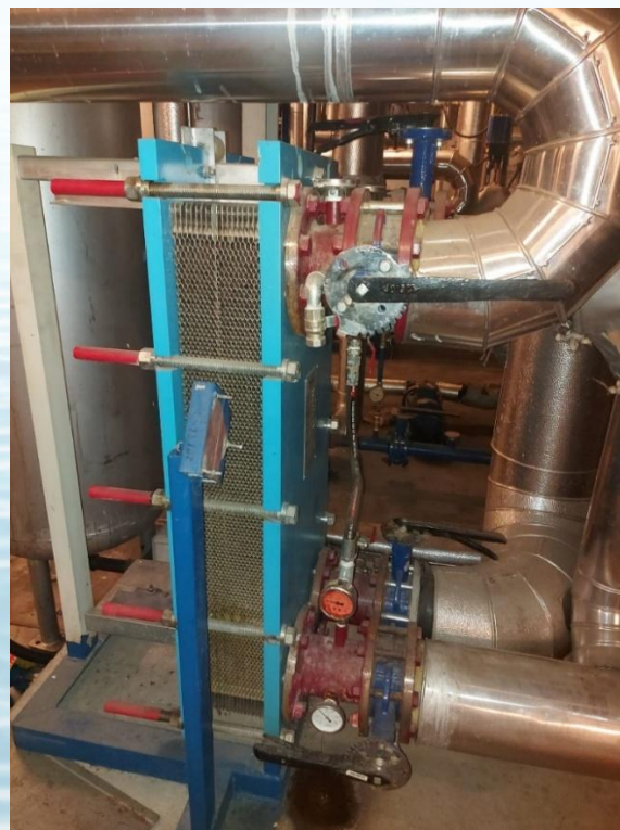
Figure 2. Jacket water-hot water heat exchanger
