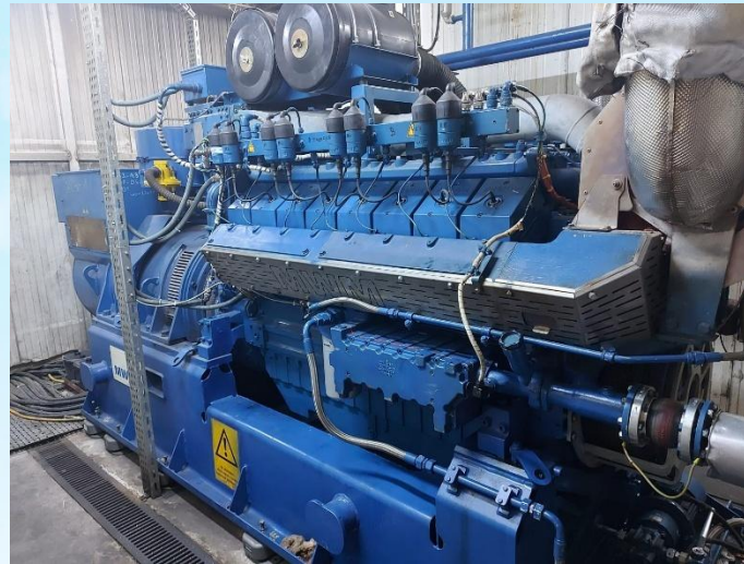
Figure 1. Natural gas-powered generator
